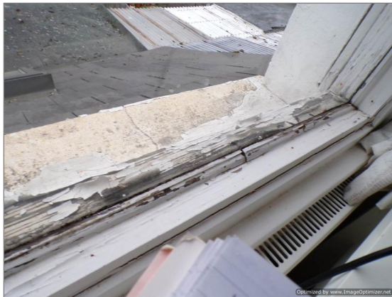
Photo - 56 Defects noted
