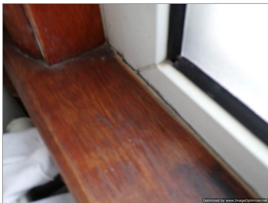
Photo - 54 Cracking/defective sealants noted
