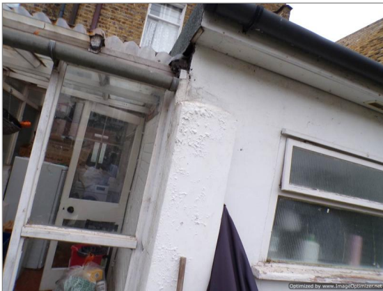
Photo - 40 Possible damp patches noted on bedroom ceiling
