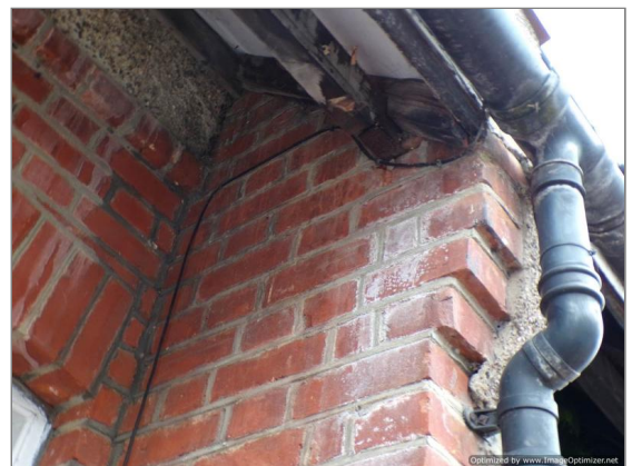
Photo - 33 Possible leak stains/defects noted
