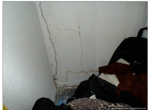
Photo - 116 Evidence of a possible structural movement/ defect/leak stains noted
