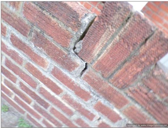
Photo - 189 Defects noted
