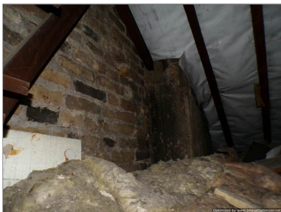
Photo - 73 Leak stains noted on chimney breast
