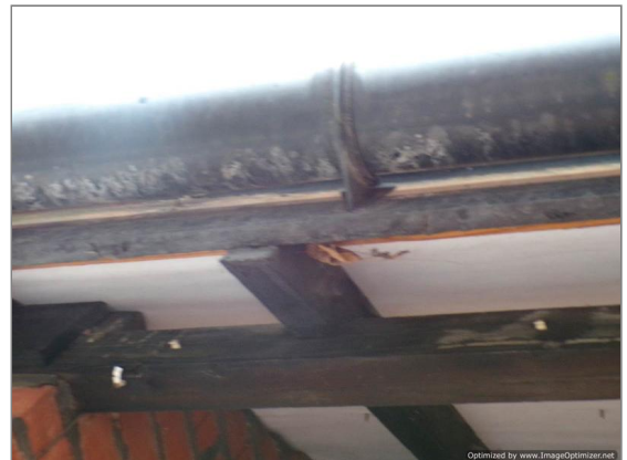
Photo - 22 Defects noted
