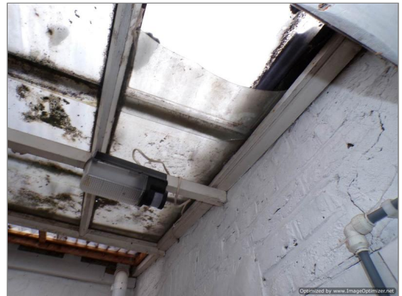
Photo - 41 Evidence of a possible structural movement/defect
