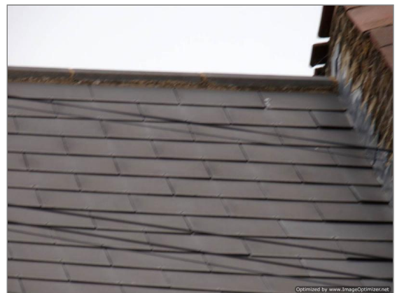
Photo - 8 Possible slipped/defective slates noted.
