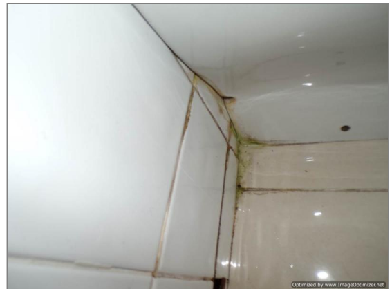
Photo - 174 Leak stains noted
