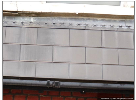
Photo - 12 Defects noted
