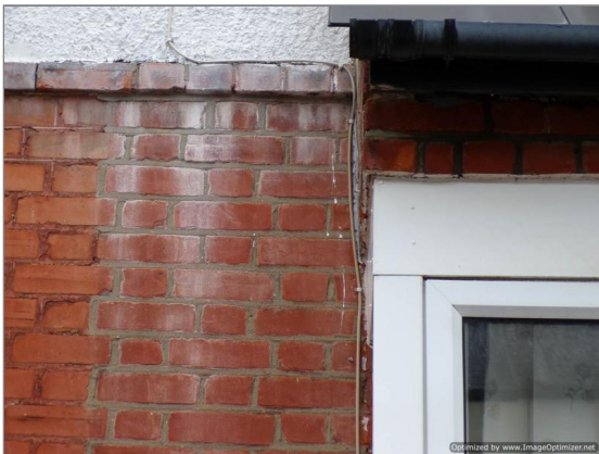
Photo - 30 Possible leak stains noted
