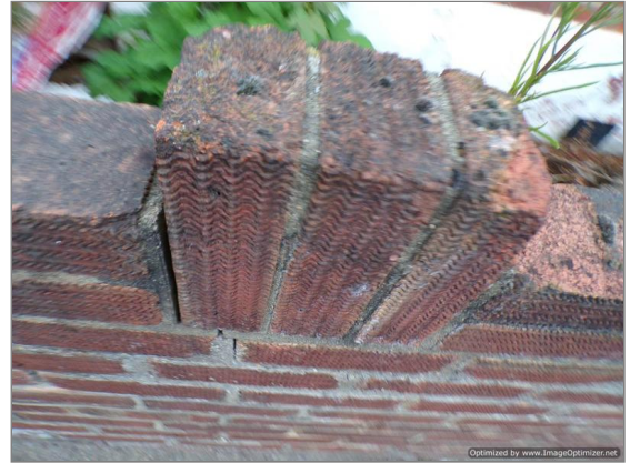
Photo - 184 Defects noted
