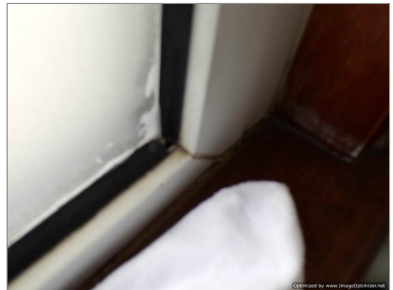
Photo - 53 Leak stains noted
