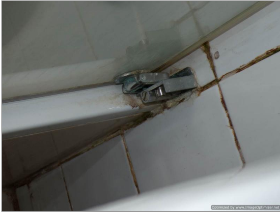
Photo - 165 Leak stains/defects noted
