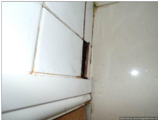
Photo - 173 Defects noted
