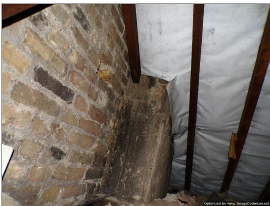
Photo - 79 Leak stains noted
