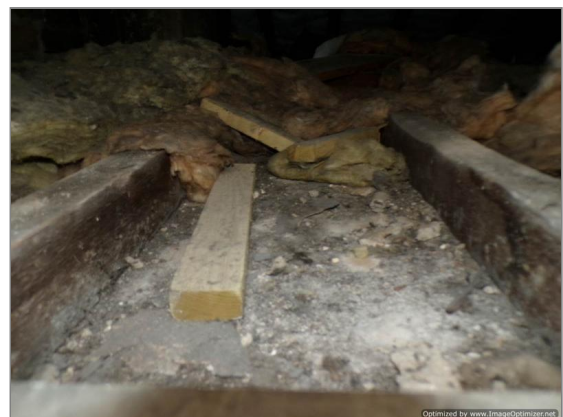
Photo - 74 Inadequate insulation noted in this area
