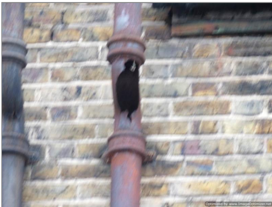
Photo - 25 Rusty and defective soil and vent pipe
