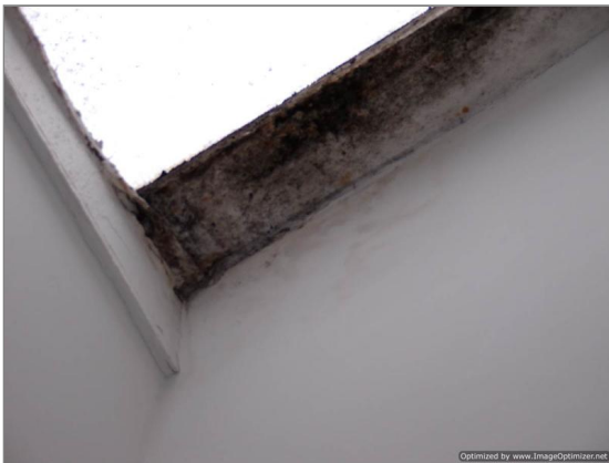
Photo - 85 Leak stains/defects noted
