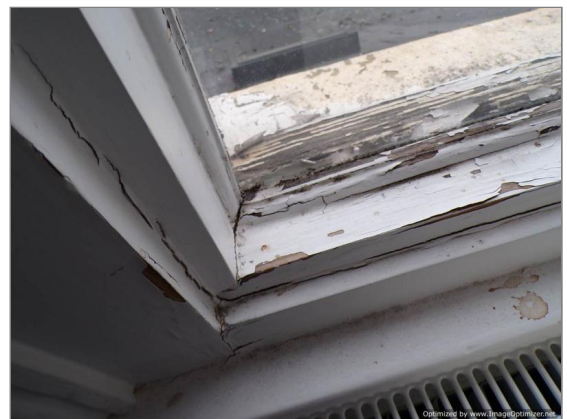
Photo - 55 Cracking/timber decay/defects on windows noted
