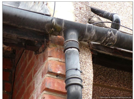
Photo - 20 Defective rainwater goods
