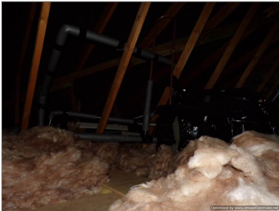
Photo - 44 Water tank noted
