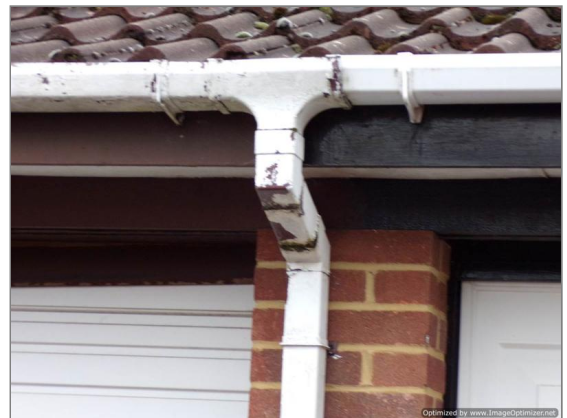
Photo - 14 Defective rainwater goods
