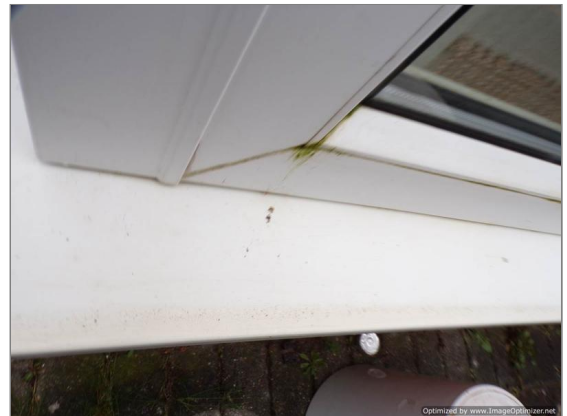
Photo - 32 Defects noted
