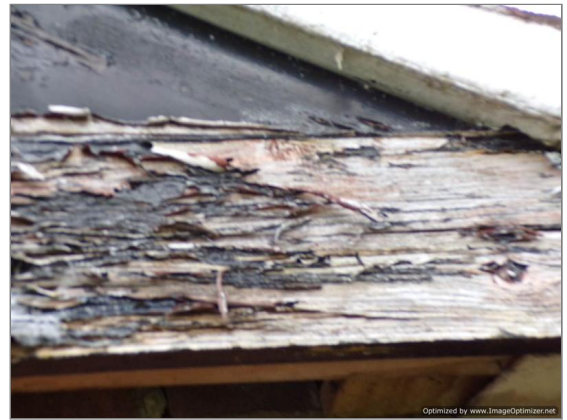
Photo - 38 Defects noted
