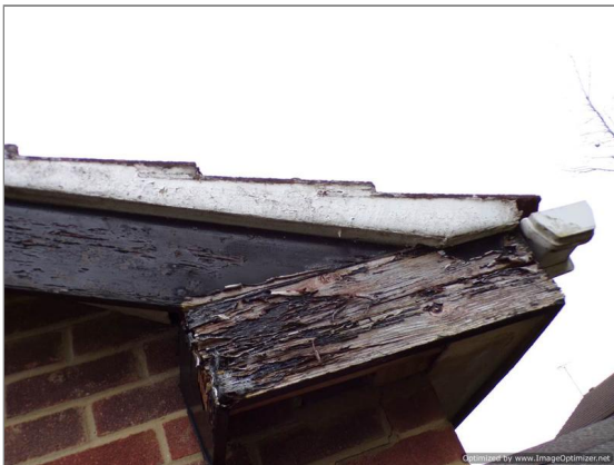
Photo - 39 Timber defect/decay noted
