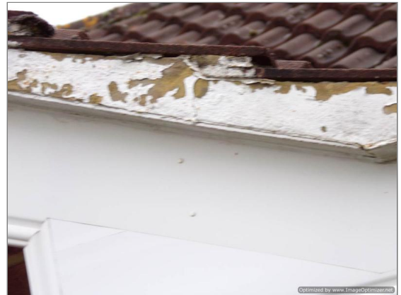
Photo - 3 Defects noted on roof verge
