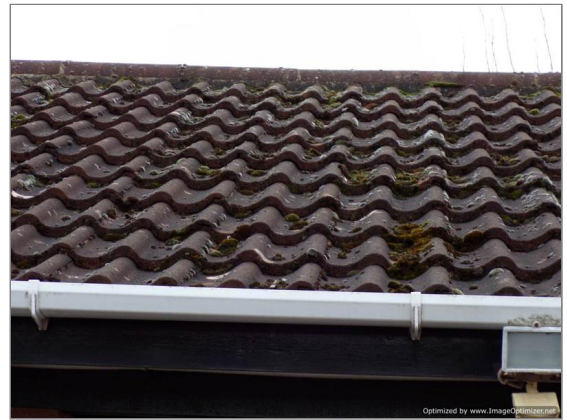
Photo - 9 Mortar pointing on ridge tiles has eroded
