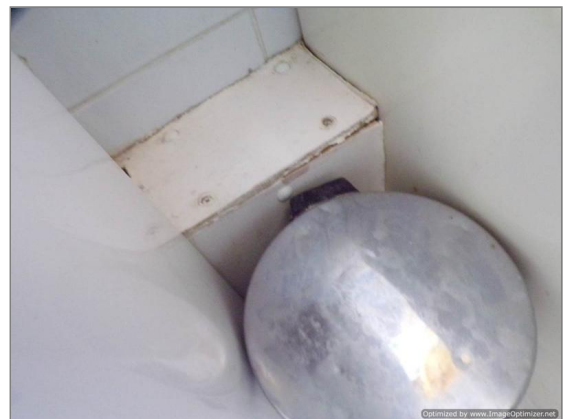
Photo - 92 Defects noted
