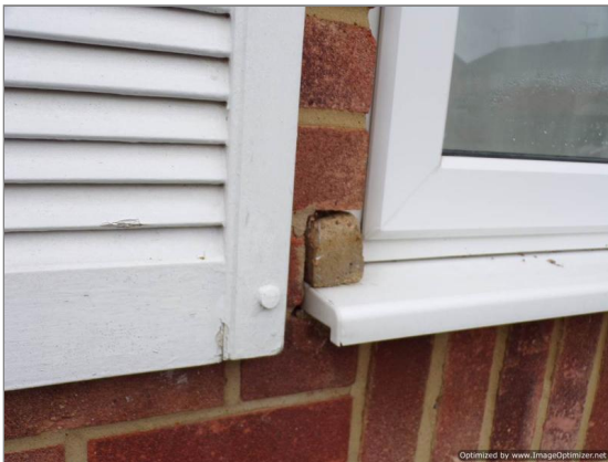
Photo - 21 Defects noted
