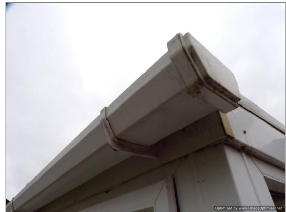
Photo - 16 Staining on the rain water goods.
