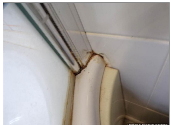
Photo - 94 Leak stains noted on shower screen.
